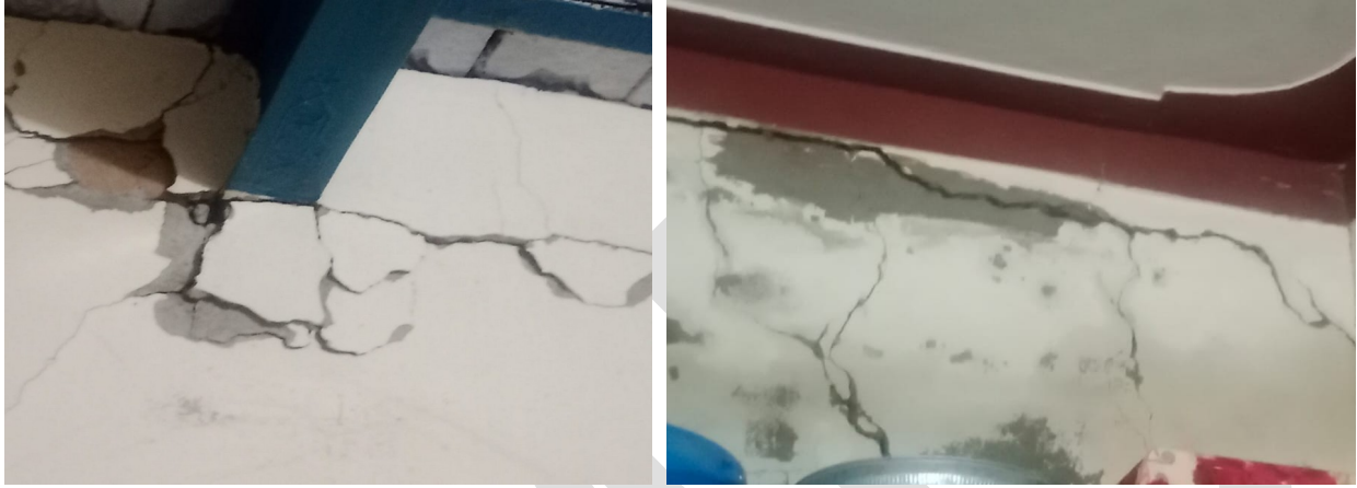
Figure 14. Field survey of a newly constructed house showing a fresh horizontal joint crack with intersecting cracks near the frame edge, representative of observations from the visual survey.
